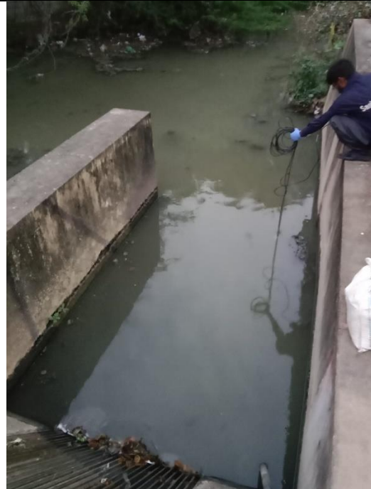
Figure 10: This image shows another view of Point 2 demarcated on Figure 1 (Identified as the STP inlet).
