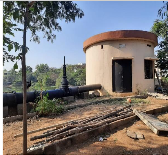
Figure 15: Sewage Pumping Station near the Lake
