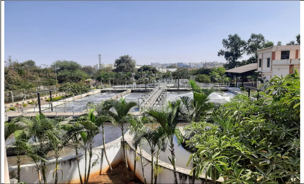
Figure 14: 5 MLD Sewage Treatment Plant (STP) established and operations along the bank of the lake
