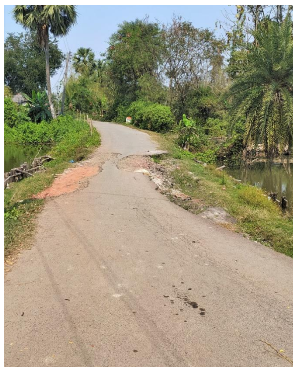
Photo 4.11: Damage of elevated village roads from flooding
