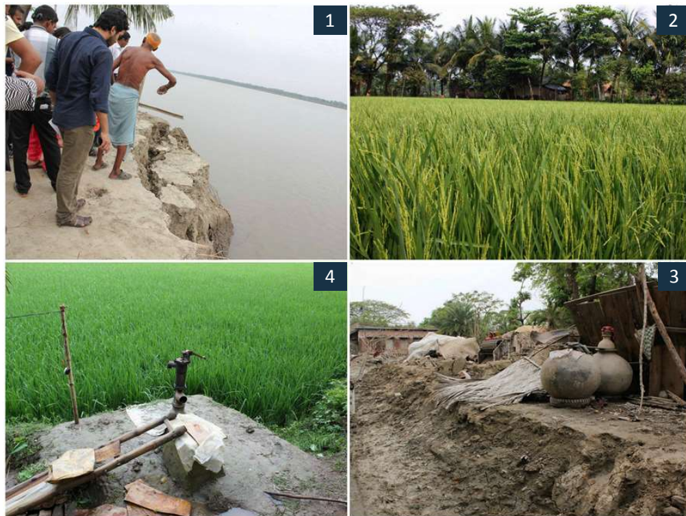
Picture 1: Erosion of a coastal riverbank in southwest Bangladesh
