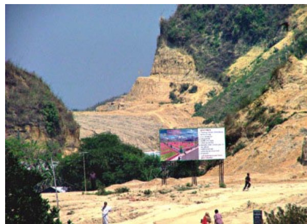
Hill cutting leading to increased soil erosion and siltation of the open drainage in the peri urban areas of Guwahati
